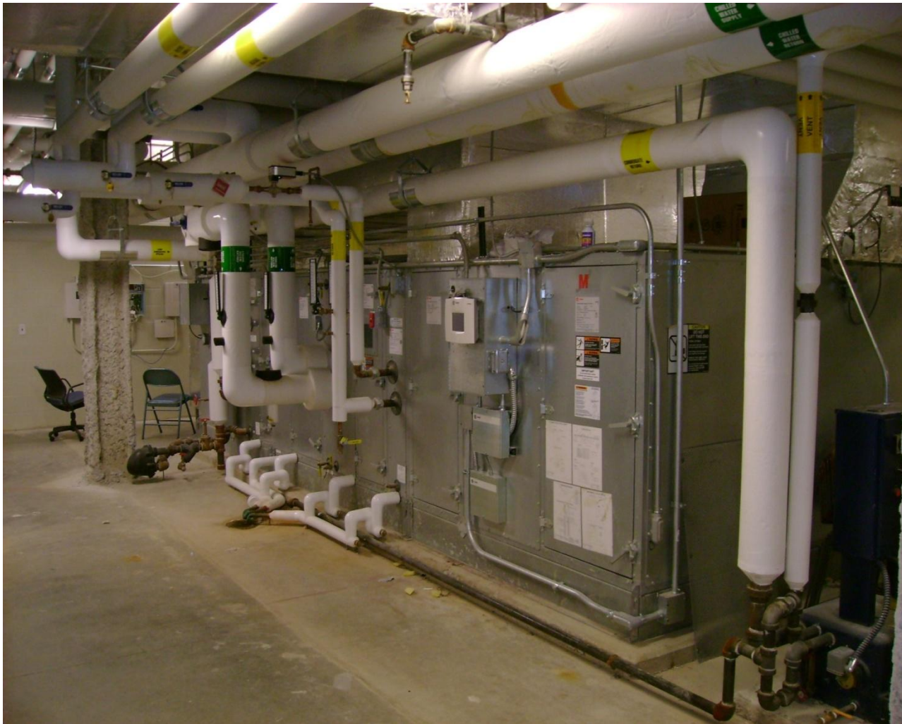
Typical Air Handling Unit Chilled Water Coil- 42 degree F water Hot Water Coil- 150 degree F water
